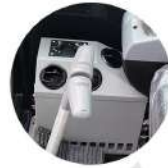
空调 Air conditioning
